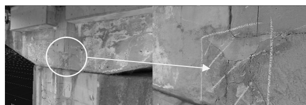
図-8 ひび割れ幅0.1～0.3mm
